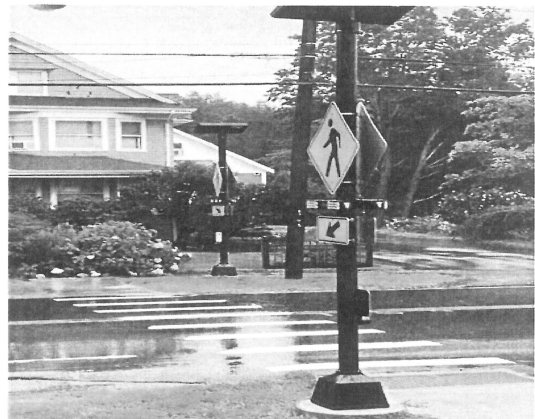
New LED Rectangular Rapid Flashing Beacons at Greenland Central School
