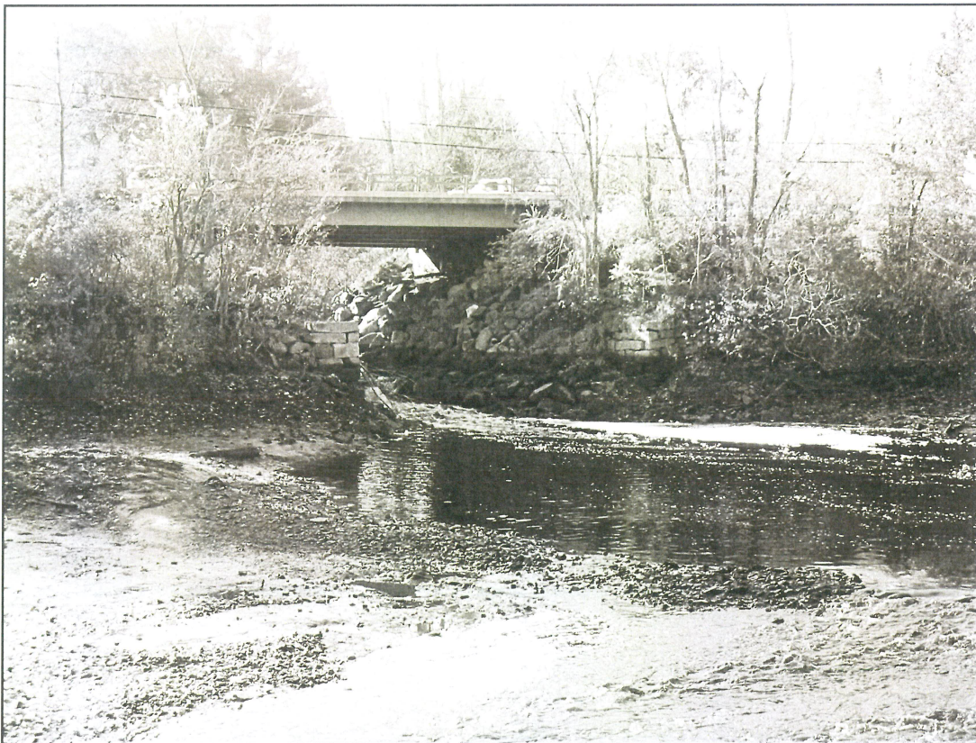
Photo Caption: The bridge that carries Route 33 over the Winnicut River in as seen in 2003, before the fish ladder was installed. Note the high-water mark left by the pond.
